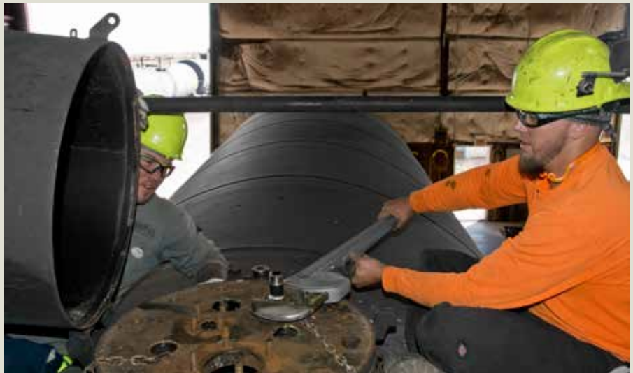
Scott Smith (left) and Lance Shumway use a 4-foot-long pipe wrench to remove a stubborn fitting atop a tank car undergoing its qualification at the Apache Railway.
